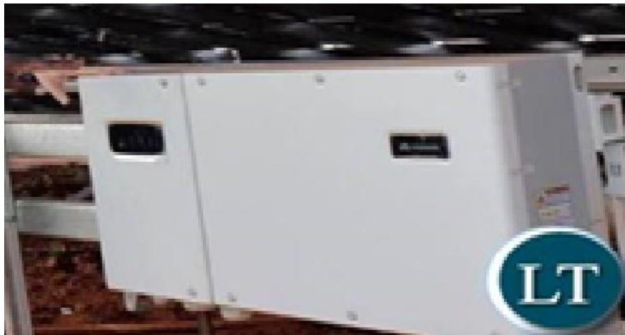
Fig. 24. Huawei - 480-volt Inverter from Bangweulu solar power station
